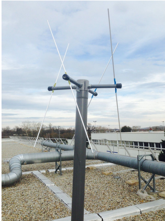
Picture of our Double-Cross antenna on the roof of Satcom's lab
